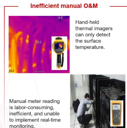
Figure 3-5 Typical manual O&M of the power supply system for a data center
